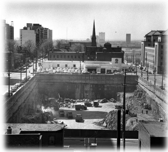
Excavation of Campeau Corporation's Place de Ville between Lyon and Kent @ Sparks St, Photo: CA023093. Thirty to forty 260-horsepower dump trucks were kept in continuous operation, hauling 6,000 tons of rock a day. To exit the pit they had to climb a vertiginous 30-degree ramp.
